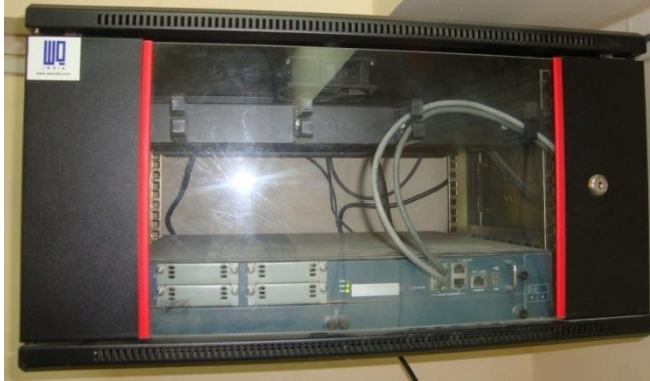
Router for internal to external connectivity
